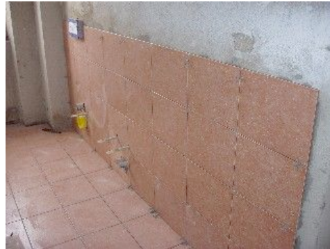
... and this is the bathroom tiling - again in our apartment - well on its way to completion.
