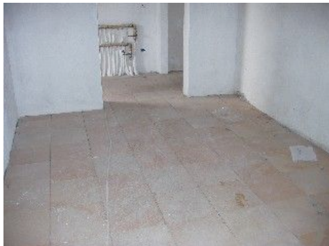
. and it's not just our apartment that is getting the floor treatment either - here is the library.
