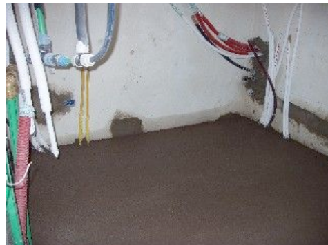
Downstairs, the boiler room floor is now 'pipeless' - the same cannot be said for the walls though!
