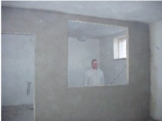
The new kitchen wall - now rough-plastered with Derek testing it out for size.
