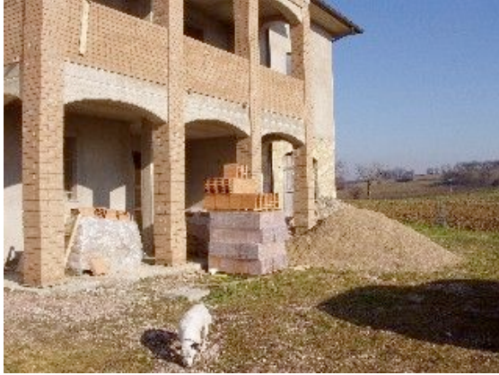
Builders materials on-site - yippee!! Josie checking for any meat scraps after the builders' lunch!
