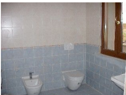
Here is the nearly finished bathroom for one of the other suites
