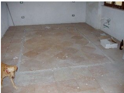
This is the floor in one of the suites, partially tiled - with Lucie just peeping in!
